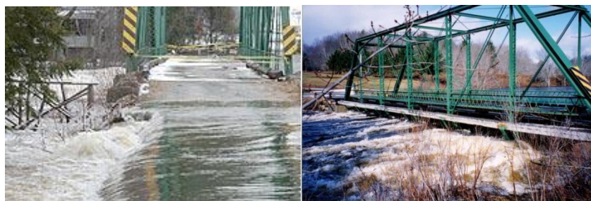
Figure 1:14 Right: The Bruhm Road Bridge on March 31, 2003. Source: http://southshorenova.ca/archives/viewer.php?sctn=2003/040903/news&article=20 (Left) Another bridge over the LaHave River during the same flood event. Source: Stan Mason.
