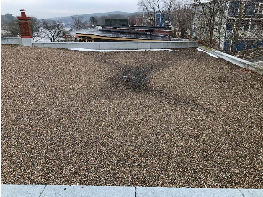
Photograph 3 – Roof drain that was considered for the existing stormwater flow estimate.
